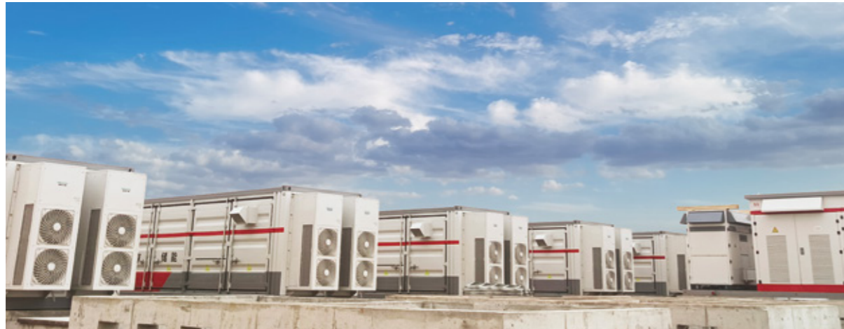
宁夏银川200MW/800MWh储能项目 200MW/800MWh Energy Storage Project in Yinchuan, Ningxia
