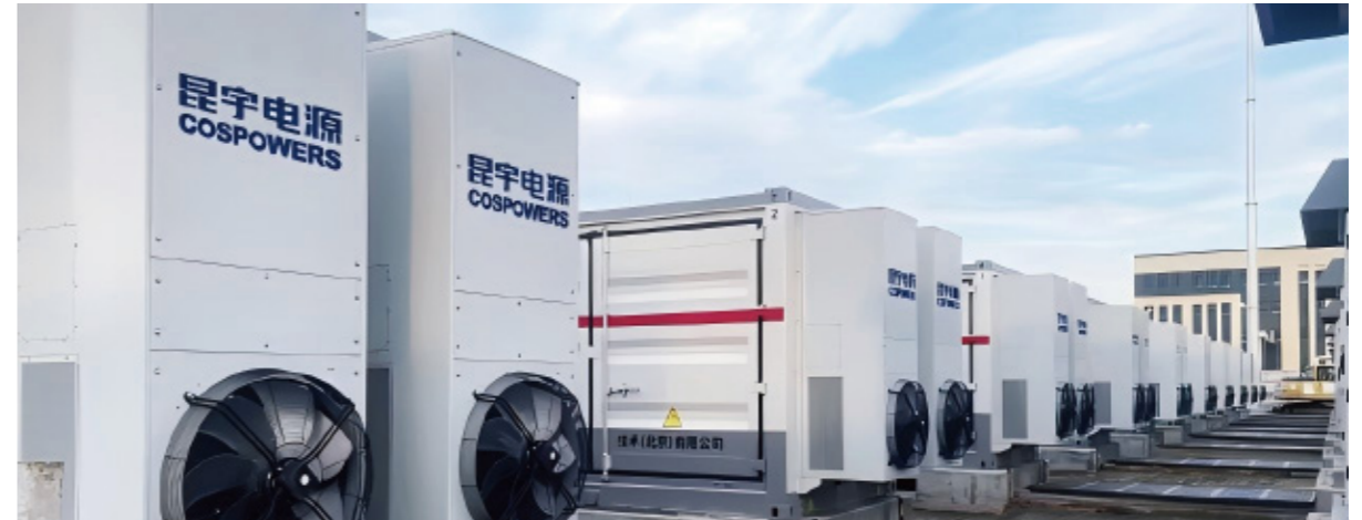
安徽天长200MW渔光互补发电87.5MW/175MWh储能项目 200MW Aquaculture-Photovoltaic Complementary Power Generation and 87.5MW/175MWh Energy Storage Project in Tianchang, Anhui
