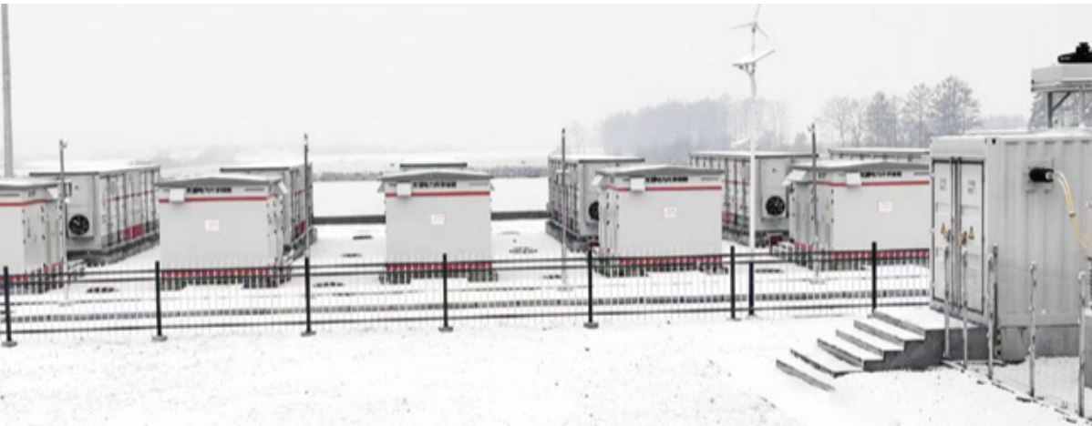
黑龙江伊春铁力年丰20MW风力发20MW/40MWh电储能项目 20MW Wind Power and 20MW/40MWh Battery Energy Storage Project in Nianfeng, Tieli, Yichun, Heilongjiang
