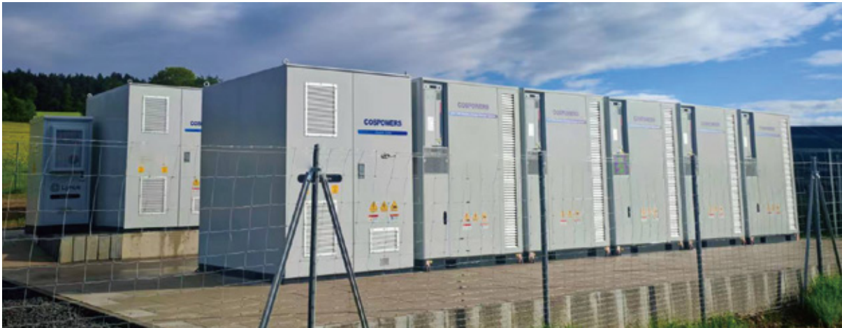
德国12MW/10.02MWh储能项目 Germany 12MW/10.02MWh Energy Storage Project
